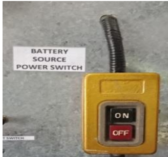
Battery source power switch
